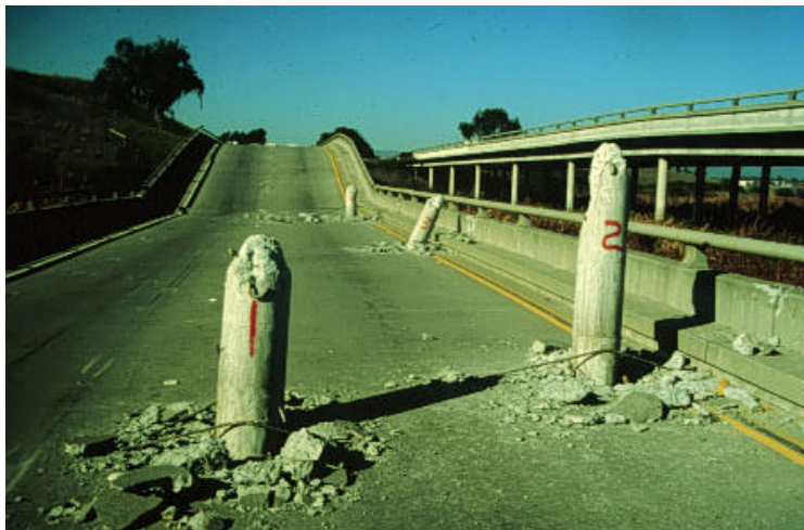
Fig. 6.4 Failure of bridge due to liquefaction, close-up view (Courtesy: http://www.es.ucsc.edu )
