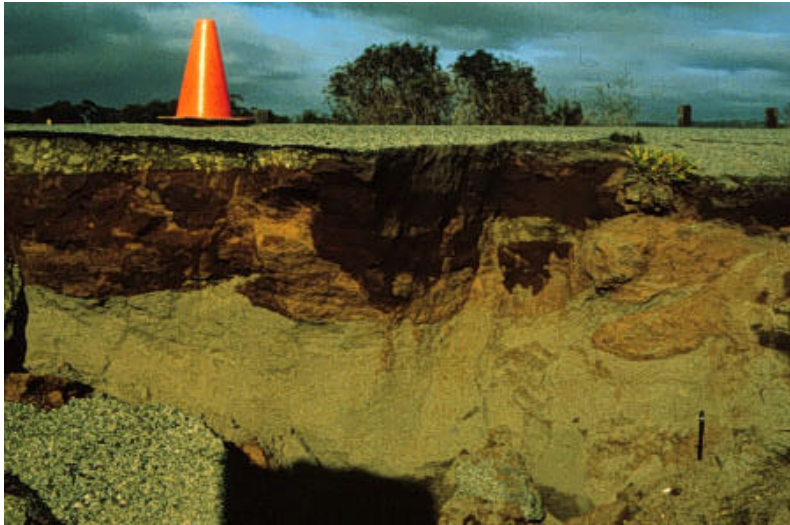
Fig. 6.6(b) Liquefaction induced road failure, exposed cross section of underlying soils (Courtesy: http://www.es.ucsc.edu )
