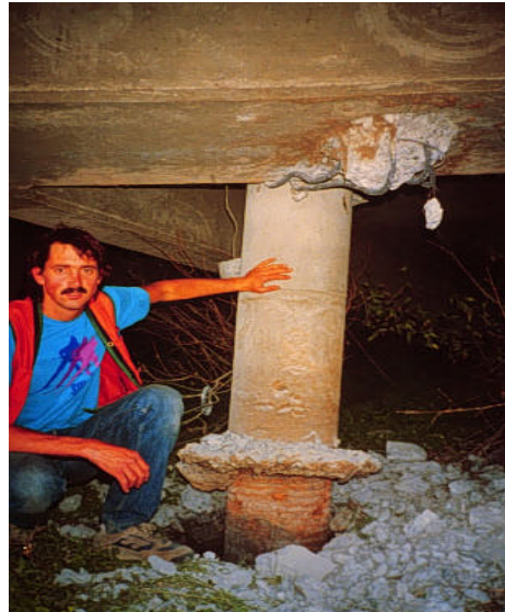
Fig. 6.5 Failure of bridge due to liquefaction, close-up view from below (Courtesy: http://www.es.ucsc.edu )
