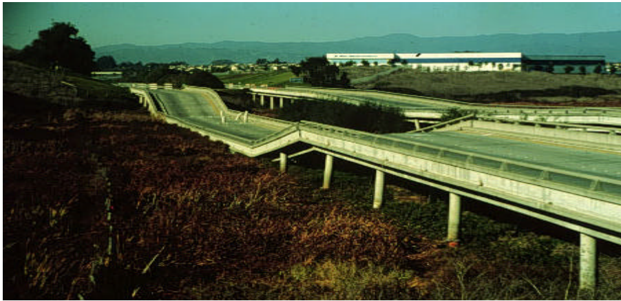
Fig. 6.3 Failure of bridge due to liquefaction (Courtesy: http://www.es.ucsc.edu )
