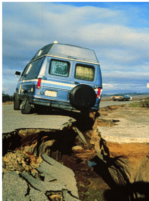
Fig. 6.6(a) Liquefaction induced road failure (Courtesy: http://www.es.ucsc.edu )
