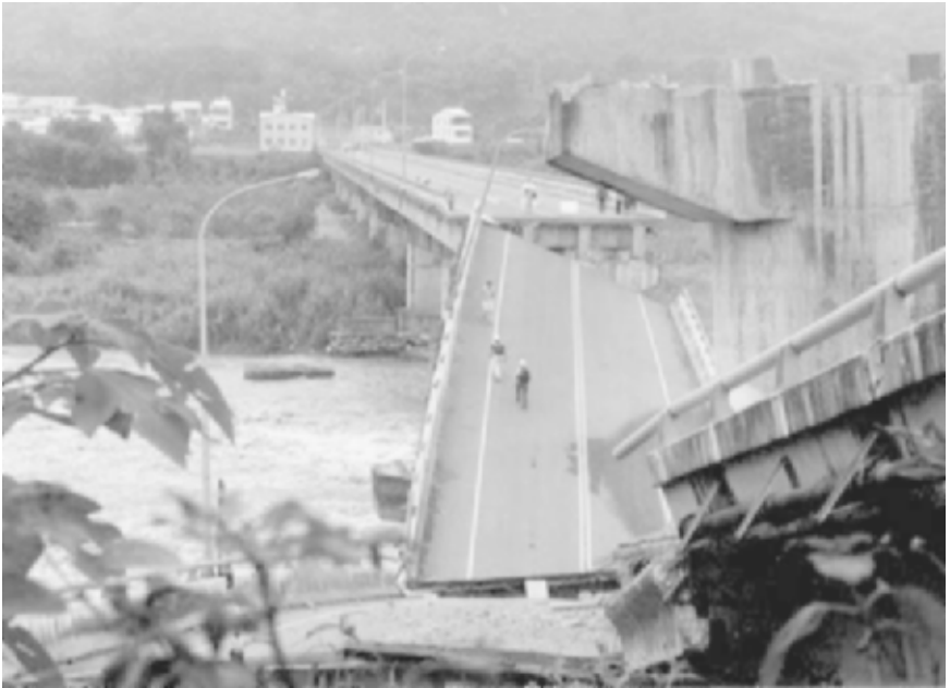
FIGURE 3.10 Another view of the collapsed bridge north of Fengyuen caused by surface fault rupture associated with the Chi-chi (Taiwan) earthquake on September 21, 1999. (Photograph from the USGS Earthquake Hazards Program, NEIC, Denver.)
