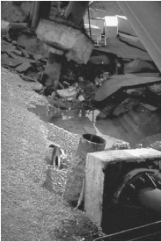
FIGURE 13.35 The top of the steel pile separated from the concrete pile cap during the Kobe earthquake on January 17, 1995. (Photograph from the Kobe Geotechnical Collection, EERC, University of California, Berkeley.)
