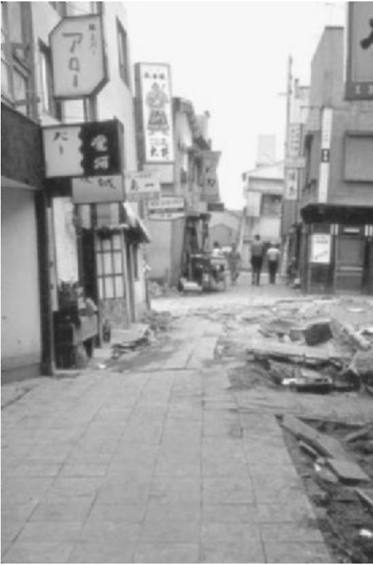
FIGURE 3.24 Settlement and tilting of relatively light buildings located in Niigata, Japan. The buildings suffered liquefaction-induced settlement and tilting during the Niigata earthquake on June 16, 1964. (Photograph from the Steinbrugge Collection, EERC, University of California, Berkeley.)
