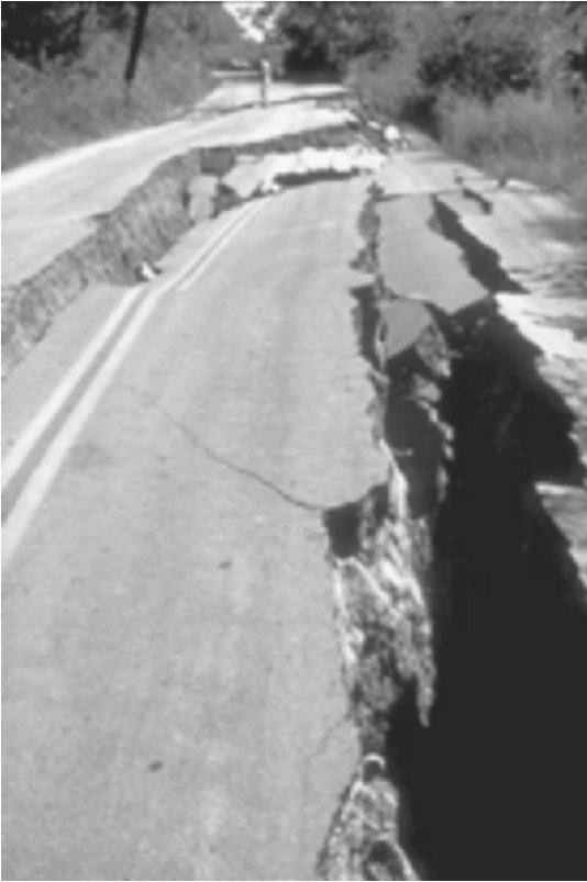
FIGURE 9.35 Earthquake damage to a two-lane road in Santa Cruz Mountains. The slope movement was caused by the Loma Prieta earthquake in California on October 17, 1989. (Photograph from the Loma Prieta Collection, EERC, University of California, Berkeley.)
