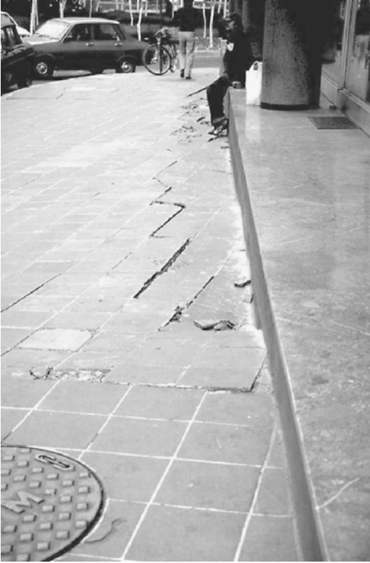
FIGURE 7.11 Settlement caused by the building rocking back and forth during the Michoacan earthquake in Mexico on September 19, 1985. (Photograph from the Steinbrugge Collection, EERC, University of California, Berkeley.)
