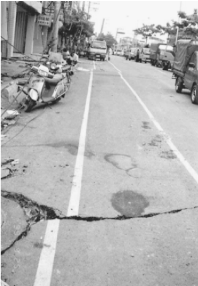
FIGURE 3.13 Surface fault rupture and roadway damage associated with the Chi-chi (Taiwan) earthquake on September 21, 1999. (Photograph from the USGS Earthquake Hazards Program, NEIC, Denver.)
