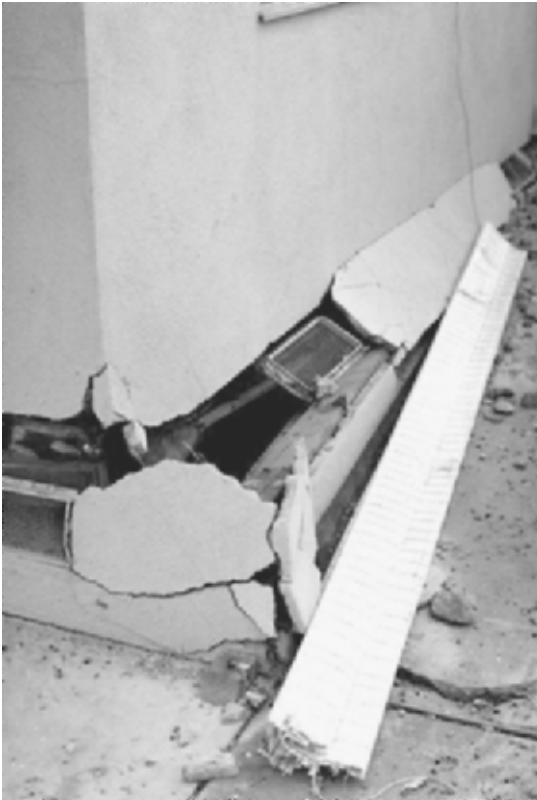
FIGURE 13.37 Sliding of house off the foundation caused by the San Fernando earthquake in California on February 9, 1971. The house is located in the city of San Fernando, near Knox and Grove Streets. (Photograph from the Steinbrugge Collection, EERC, University of California, Berkeley.)
