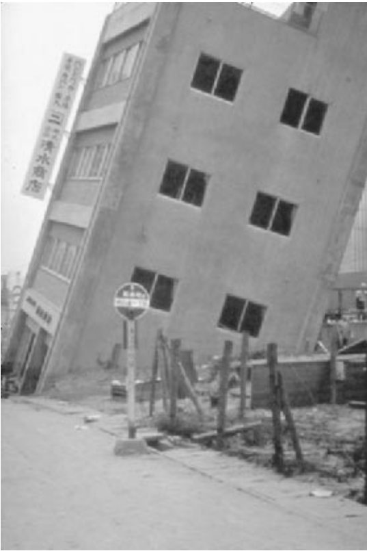
FIGURE 3.23 Settlement and tilting of a building located in Niigata, Japan. The building suffered liquefaction-induced settlement and tilting during the Niigata earthquake on June 16, 1964. (Photograph from the Steinbrugge Collection, EERC, University of California, Berkeley.)
