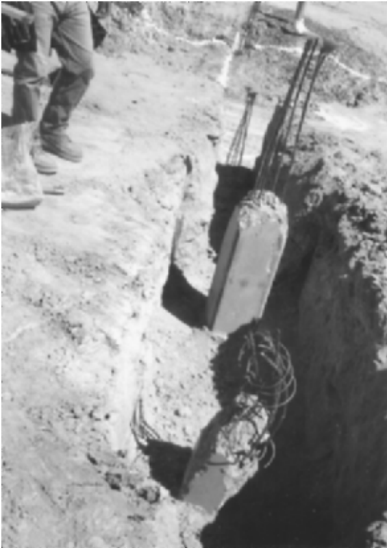
FIGURE 13.30 The prestressed concrete pile at the bottom of the picture is the same pile shown in Figure 13.23. The pile near the center of the photograph is the replacement pile. The broken pile and the replacement pile will be attached to the grade beam.
