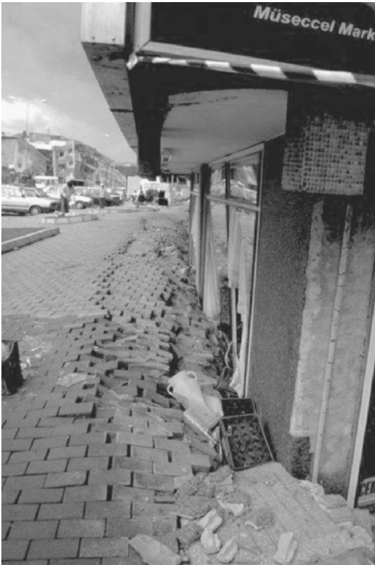
FIGURE 8.5 The building suffered a liquefaction-induced punching shear failure during the Izmit earthquake in Turkey on August 17, 1999. (Photograph from the Izmit Collection, EERC, University of California, Berkeley.)
