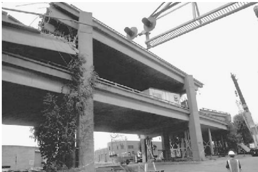
FIGURE 4.29 Close-up view of the collapse of the Cypress Street Viaduct caused by the Loma Prieta earthquake in California on October 17, 1989. (From USGS.)
