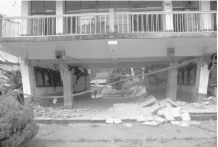
FIGURE 3.6 Portion of a building that remained standing at the Kuang Fu Elementary School. This portion of the building was directly adjacent to the surface fault rupture associated with the Chi-chi (Taiwan) Earthquake on September 21, 1999. Note in this figure that the ground was actually compressed together adjacent to the footwall side of the fault rupture. (Photograph from the Taiwan Collection, EERC, University of California, Berkeley.)
