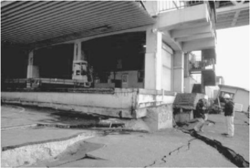
FIGURE 3.35 Settlement caused by lateral movement of a retaining wall during the Kobe earthquake on January 17, 1995. The industrial building is supported by a pile foundation. The Higashi Kobe cable-stayed bridge is visible in the upper right corner of the photograph. (Photograph from the Great Hanshin Bridge Collection, EERC, University of California, Berkeley.)
