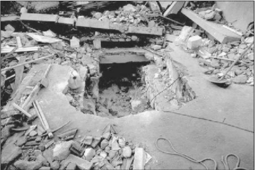
FIGURE 4.16 Pancaking of a building, during the Izmit earthquake in Turkey on August 17, 1999. Note that the center of the photograph shows a hole that was excavated through the pancaked building in order to rescue the survivors. (Photograph from the Izmit Collection, EERC, University of California, Berkeley.)
