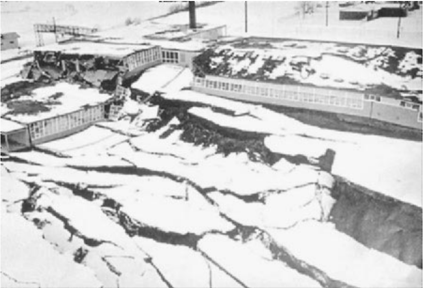
FIGURE 3.52 Overview of damage to the Government Hill School located at the head of a landslide caused by the Prince William Sound earthquake in Alaska on March 27, 1964. (Photograph from the Steinbrugge Collection, EERC, University of California, Berkeley.)
