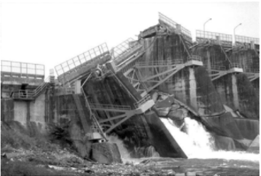
FIGURE 3.4 Close-up view of the location of the dam damaged by surface fault rupture associated with the Chi-chi (Taiwan) earthquake on September 21, 1999. Note in this figure that the entire length of fence on the top of the dam was initially at the same elevation prior to the earthquake. (Photograph from the Taiwan Collection, EERC, University of California, Berkeley.)
