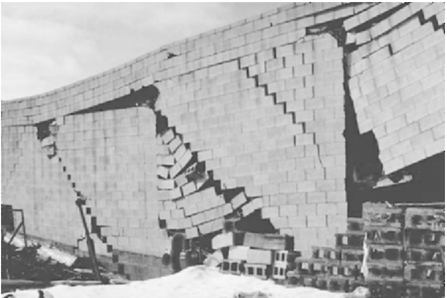
FIGURE 9.37 Building damage caused by the Fourth Avenue landslide, Anchorage, Alaska. The landslide movement occurred during the Prince William Sound earthquake in Alaska on March 27, 1964. (Photograph from the Steinbrugge Collection, EERC, University of California, Berkeley.)
