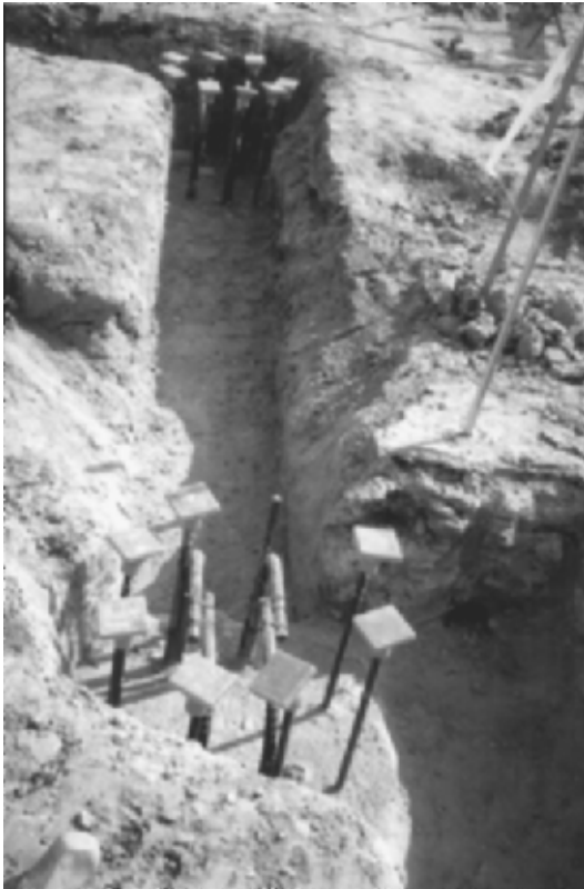
FIGURE 13.11 Excavation for the grade beam that will span between the two piers.
