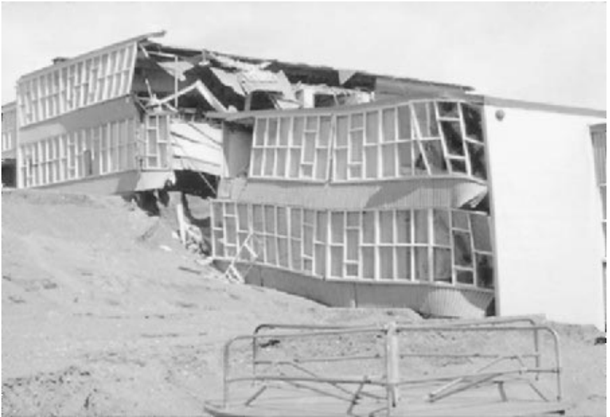
FIGURE 3.53 Close-up view of damage to the Government Hill School located at the head of a landslide caused by the Prince William Sound earthquake in Alaska on March 27, 1964. (Photograph from the Steinbrugge Collection, EERC, University of California, Berkeley.)
