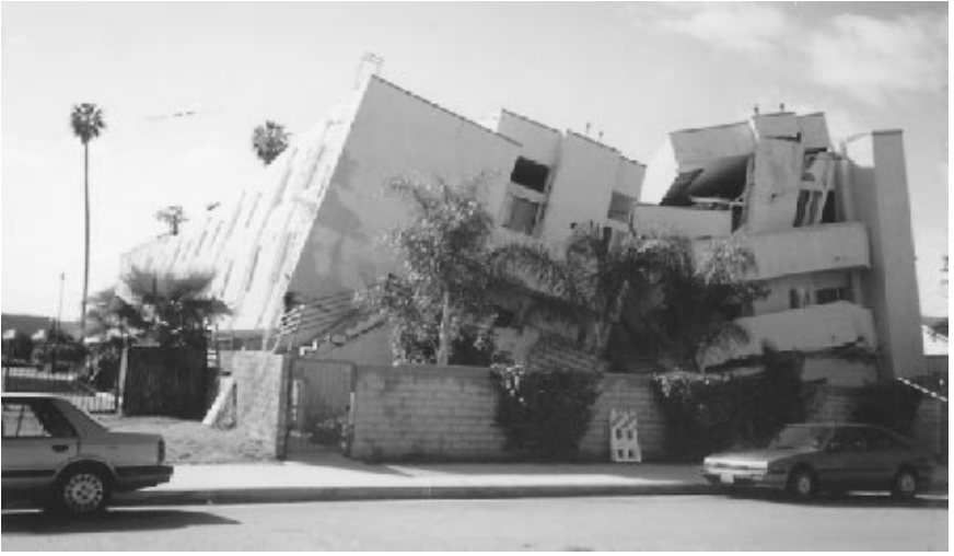
FIGURE 4.6 Building collapse caused by a soft story due to the parking garage on the first floor. The building collapse occurred during the Northridge earthquake in California on January 17, 1994.
