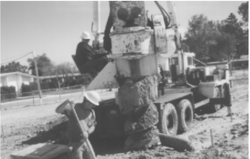
FIGURE 13.8 Close-up of auger being extracted from the ground with soil lodged within its grooves.
