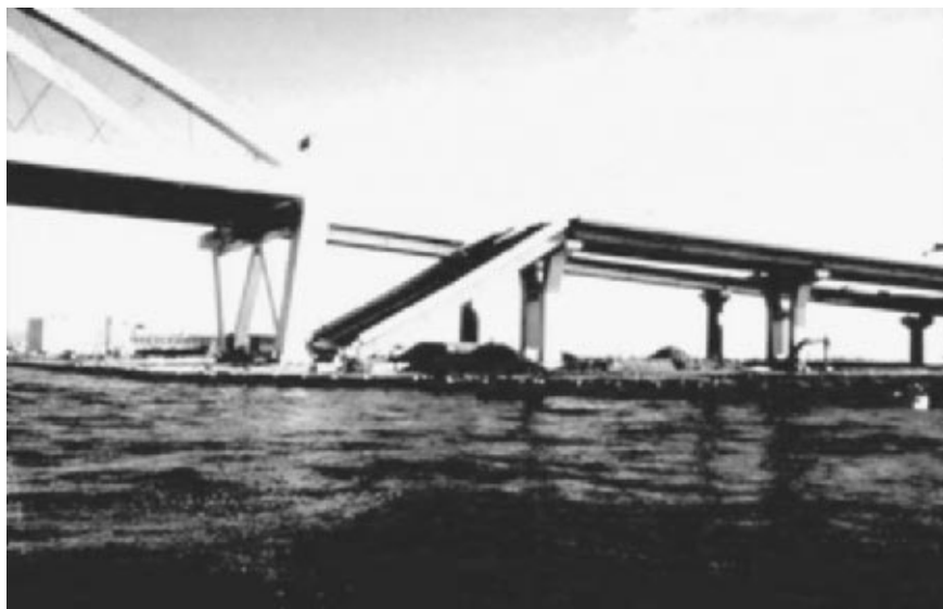
FIGURE 3.37 Collapse of a span of the Nishihomiya Bridge, apparently due to lateral retaining wall movement during the Kobe earthquake on January 17, 1995. (Photograph from the Kobe Geotechnical Collection, EERC, University of California, Berkeley.)
