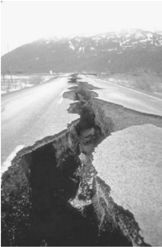
FIGURE 3.54 Cracking of the Anchorage-Portage highway. The small highway embankment experienced lateral movement during the Prince William Sound earthquake in Alaska on March 27, 1964. (Photograph from the Steinbrugge Collection, EERC, University of California, Berkeley.)
