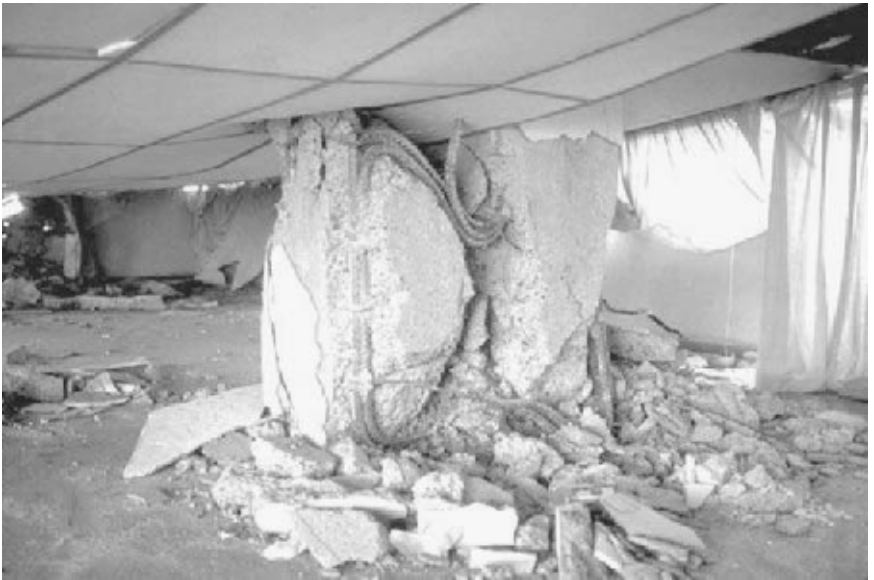
FIGURE 4.4 Close-up view of a collapsed second-story column at the Hotel Terminal. Note that the upper floor has displaced to the right and dropped, and the top and bottom sections of the column are now side by side. The torsional failure occurred during the Gualan earthquake in Guatemala on February 4, 1976. (Photograph from the Godden Collection, EERC, University of California, Berkeley.)
