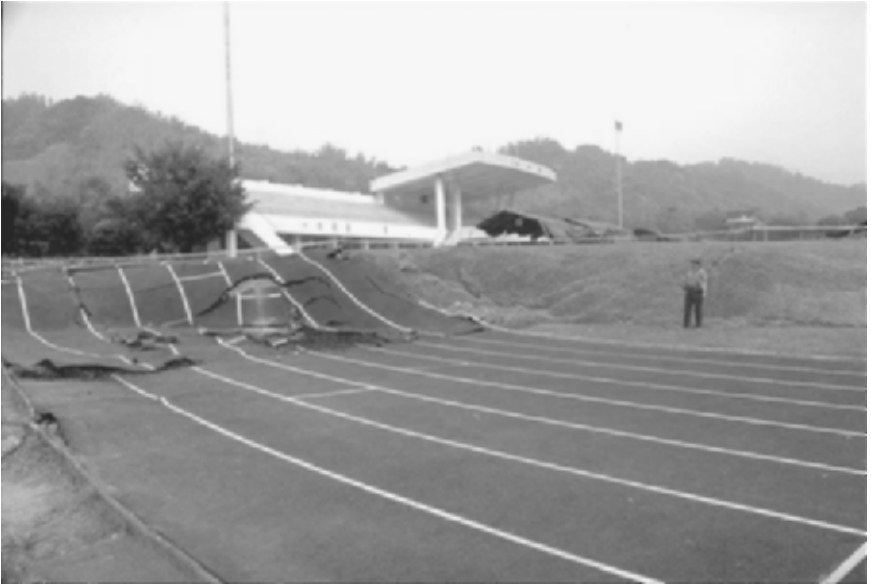
FIGURE 3.5 Overview of damage to the Kuang Fu Elementary School by surface fault rupture associated with the Chi-chi (Taiwan) earthquake on September 21, 1999. (Photograph from the Taiwan Collection, EERC, University of California, Berkeley.)
