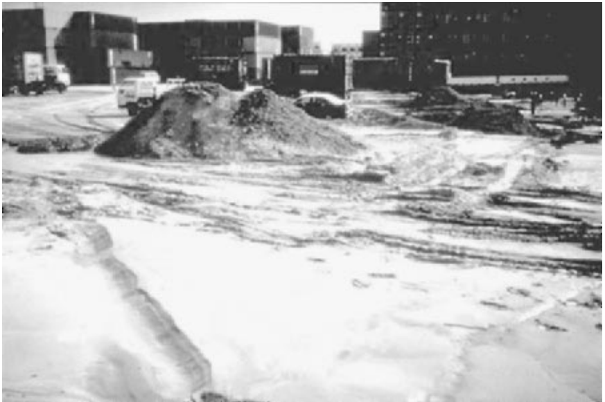
FIGURE 3.26 The interiors of the Rokko and Port islands settled as much as 1 m with an average of about 0.5 m due to liquefaction caused by the Kobe earthquake on January 17, 1995. This liquefaction-induced settlement was accompanied by the eruption of large sand boils that flooded many areas and covered much of the island with sand boil deposits as thick as 0.5 m. In this photograph, a stockpile has been created out of some of this sand. (Photograph from the Kobe Geotechnical Collection, EERC, University of California, Berkeley.)
