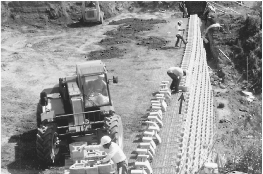
FIGURE 10.6 Installation of a mechanically stabilized earth retaining wall. The arrow points to the wall facing elements, which are in the process of being installed.
