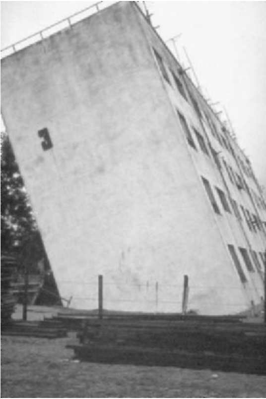
FIGURE 3.22 Settlement and tilting of an apartment building located in Niigata, Japan. The building suffered liquefaction-induced settlement and tilting during the Niigata earthquake on June 16, 1964. (Photograph from the Steinbrugge Collection, EERC, University of California, Berkeley.)
