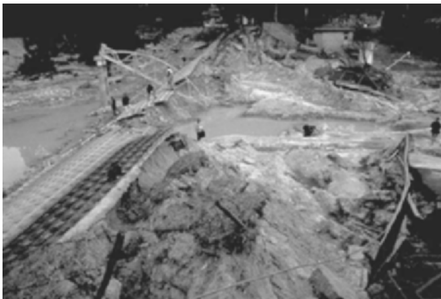
FIGURE 9.23 Flow slide of the Middle Nitoko Dam caused by the Kobe earthquake, in Japan, on January 17, 1995. (Photograph from the Kobe Geotechnical Collection, EERC, University of California, Berkeley.)
