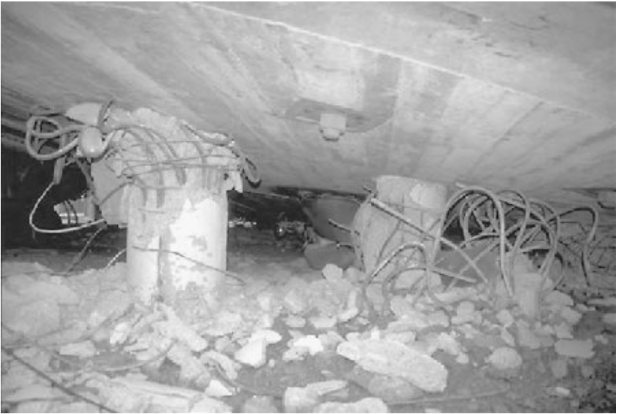
FIGURE 4.13 Close-up view of the columns that had supported the elevated gas storage tank shown in Fig. 4.12. The columns did not have adequate shear resistance and were unable to support the gas storage tank during the Izmit earthquake in Turkey on August 17, 1999. (Photograph from the Izmit Collection, EERC, University of California, Berkeley.)
