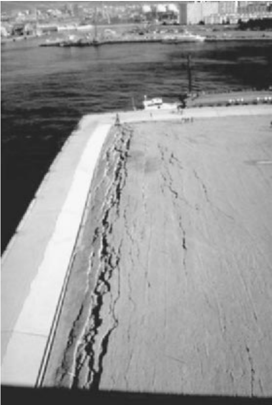
FIGURE 3.36 The liquefaction-induced retaining wall movement was caused by the Kobe Earthquake on January 17, 1995. Both lateral spreading fissures and sporadic sand boils were observed behind the retaining wall. The site is near the pier of Nishihomiya Bridge, which previously supported the collapsed expressway section. (Photograph from the Kobe Geotechnical Collection, EERC, University of California, Berkeley.)
