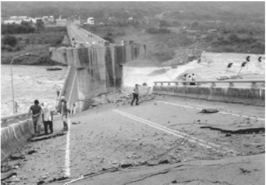
FIGURE 3.11 Another view of the collapsed bridge north of Fengyuen caused by surface fault rupture associated with the Chi-chi (Taiwan) earthquake on September 21, 1999. Note that the surface faulting has created the waterfall on the right side of the bridge. (Photograph from the USGS Earthquake Hazards Program, NEIC, Denver.)
