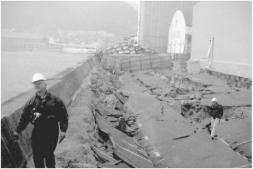
FIGURE 3.28 Lateral retaining wall movement due to liquefaction during the Kobe earthquake on January 17, 1995. As the retaining wall has moved outward, the ground surface has dropped. The site is adjacent to the east end of the Higashi Kobe Bridge. (Photograph from the Great Hanshin Bridge Collection, EERC, University of California, Berkeley.)
