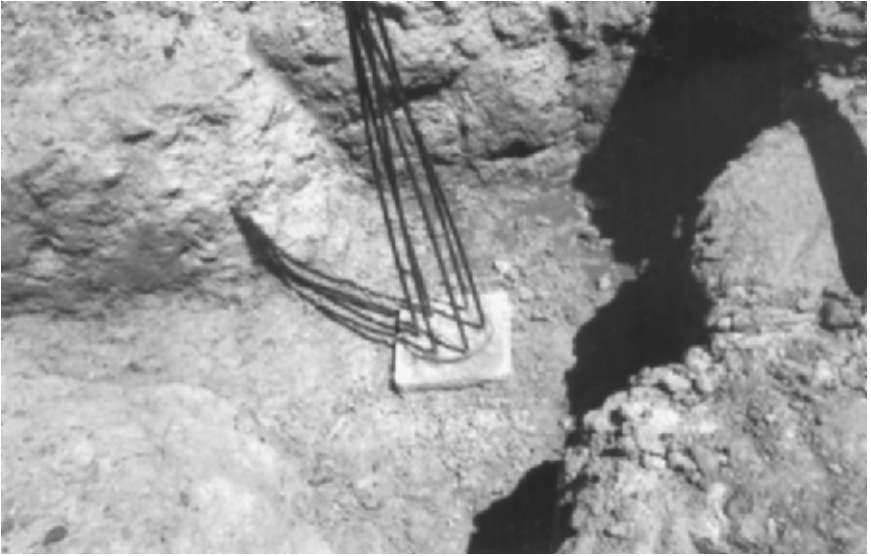
FIGURE 13.32 Close-up view of one of the prestressed piles showing a trimmed top surface with the strands extending out the top of the pile.
