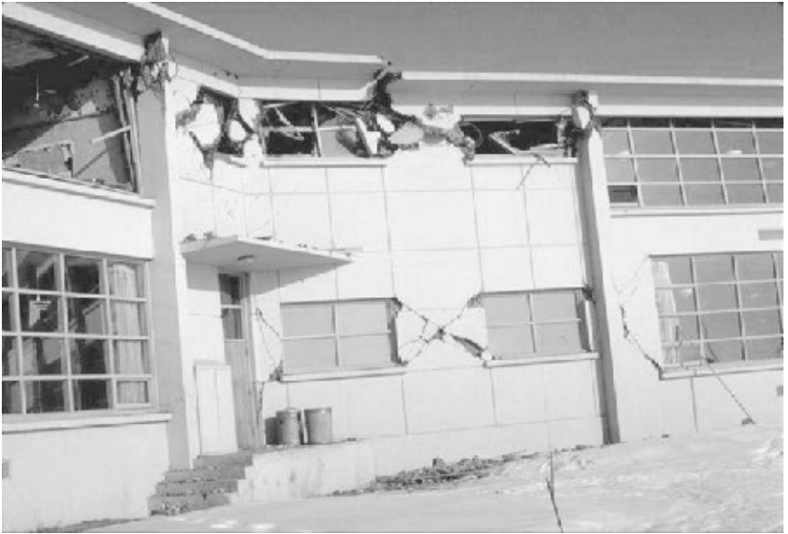
FIGURE 4.18 Damage to a shear wall at the West Anchorage High School caused by the Prince William Sound earthquake in Alaska on March 27, 1964. (Photograph from the Steinbrugge Collection, EERC, University of California, Berkeley.)
