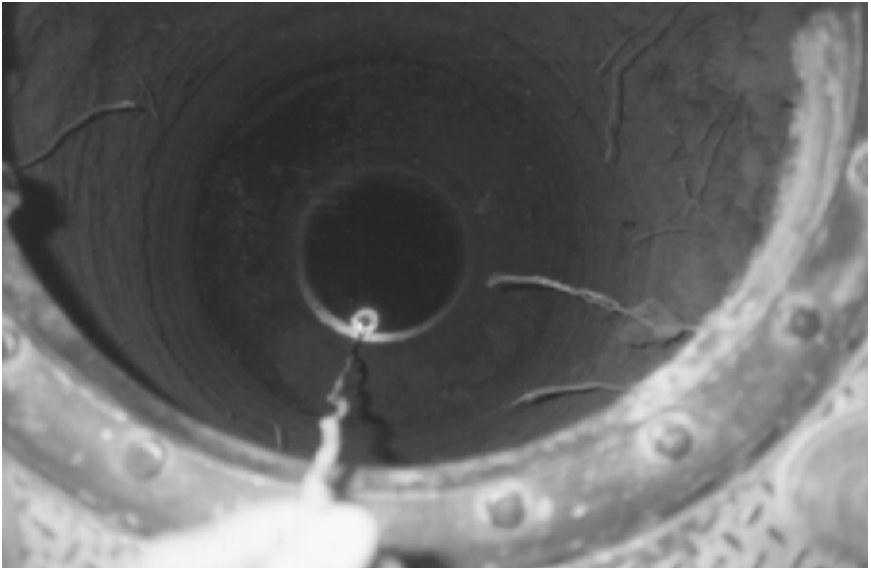
FIGURE 13.9 A light has been lowered to the bottom of the pier to observe embedment conditions.
