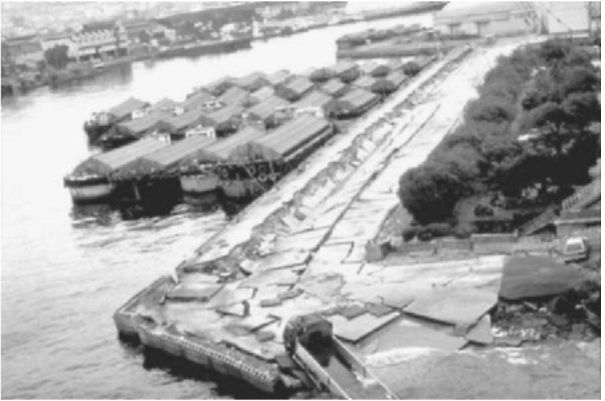
FIGURE 3.30 Retaining wall damage caused by the Kobe earthquake on January 17, 1995. The site is the east bank of the Maya-ohashi Bridge (Harbor Expressway). Liquefaction caused significant lateral displacement of the retaining wall, which in turn created a depression behind the wall and dropped a large truck halfway into the water. (Photograph from the Kobe Geotechnical Collection, EERC, University of California, Berkeley.)
