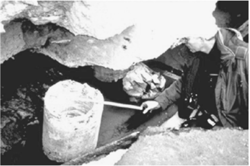
FIGURE 13.36 The top of the concrete pile separated from the concrete pile cap during the Kobe earthquake on January 17, 1995. (Photograph from the Kobe Geotechnical Collection, EERC, University of California, Berkeley.)
