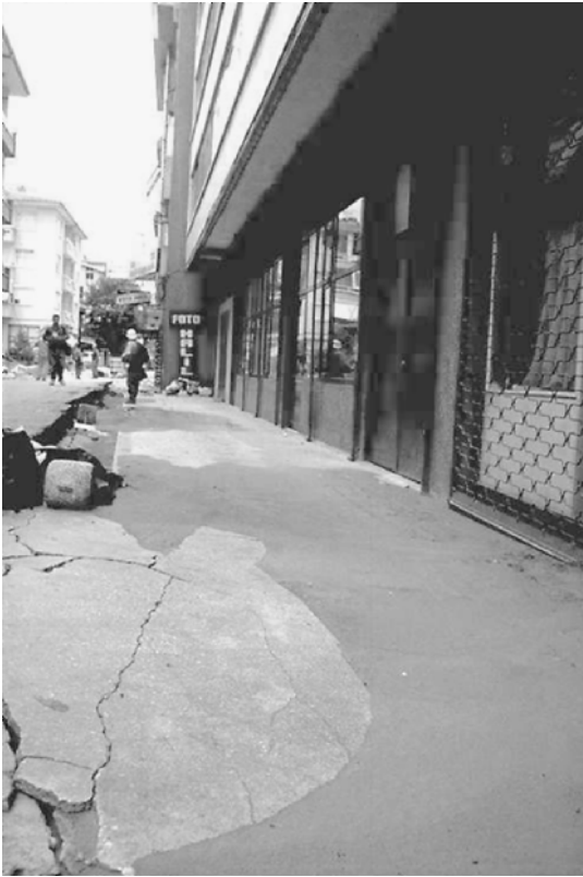
FIGURE 7.5 Surface fissure caused by the Izmit earthquake in Turkey on August 17, 1999. Note that liquefied soil flowed out of the fissure. (Photograph from the Izmit Collection, EERC, University of California, Berkeley.)
